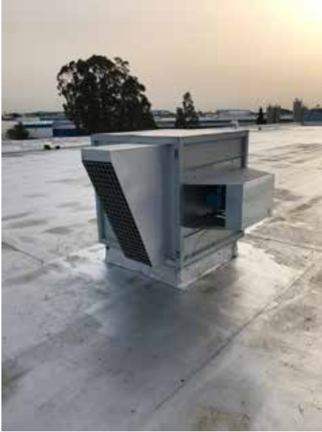
Smoke extraction in restaurant kitchen (Portugal) DHUMAT
